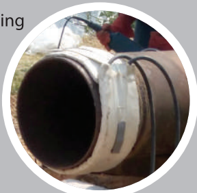
Pipe Line Heating
